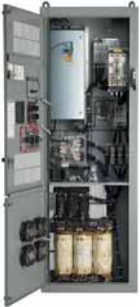
Enclosed 18-Pulse Drive
